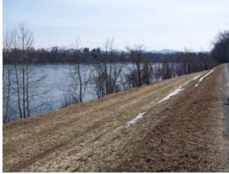
Dike along Connecticut River, 2009.
